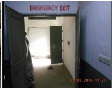
Non-compliance: Inward opening door + no emergency light
