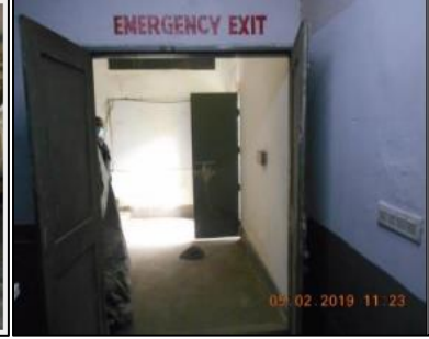
Non-compliance: Inward opening door + no emergency light 内开门+ 无应急灯
