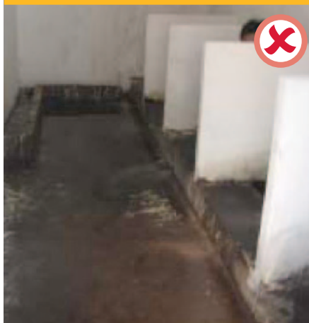
Poor factory toilet facilities
